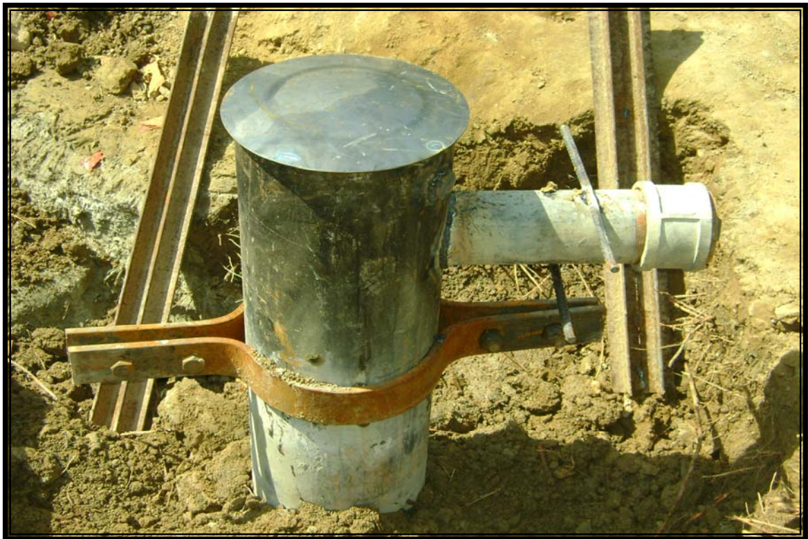
Tubewell with clamp, girders & cap
